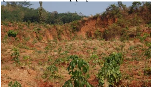
Figure 5: Arcuate failure in the Vallankolli
